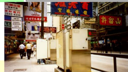
Roadside monitoring station
